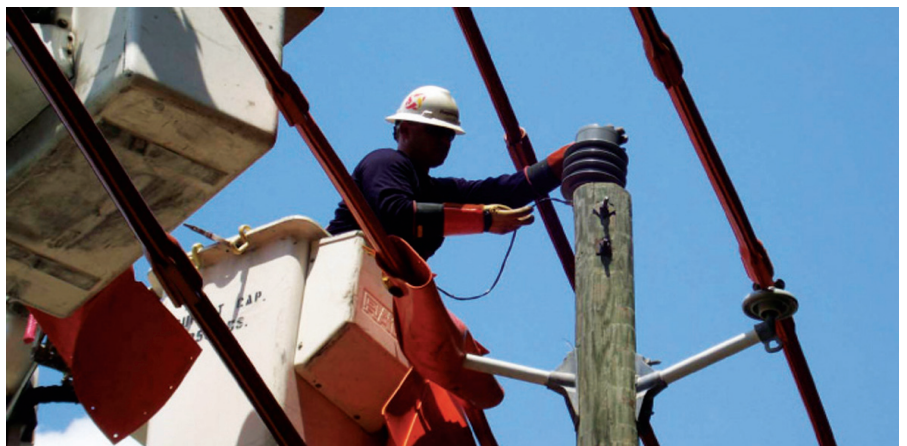
Live installation of SATEC’s Smart Grid
